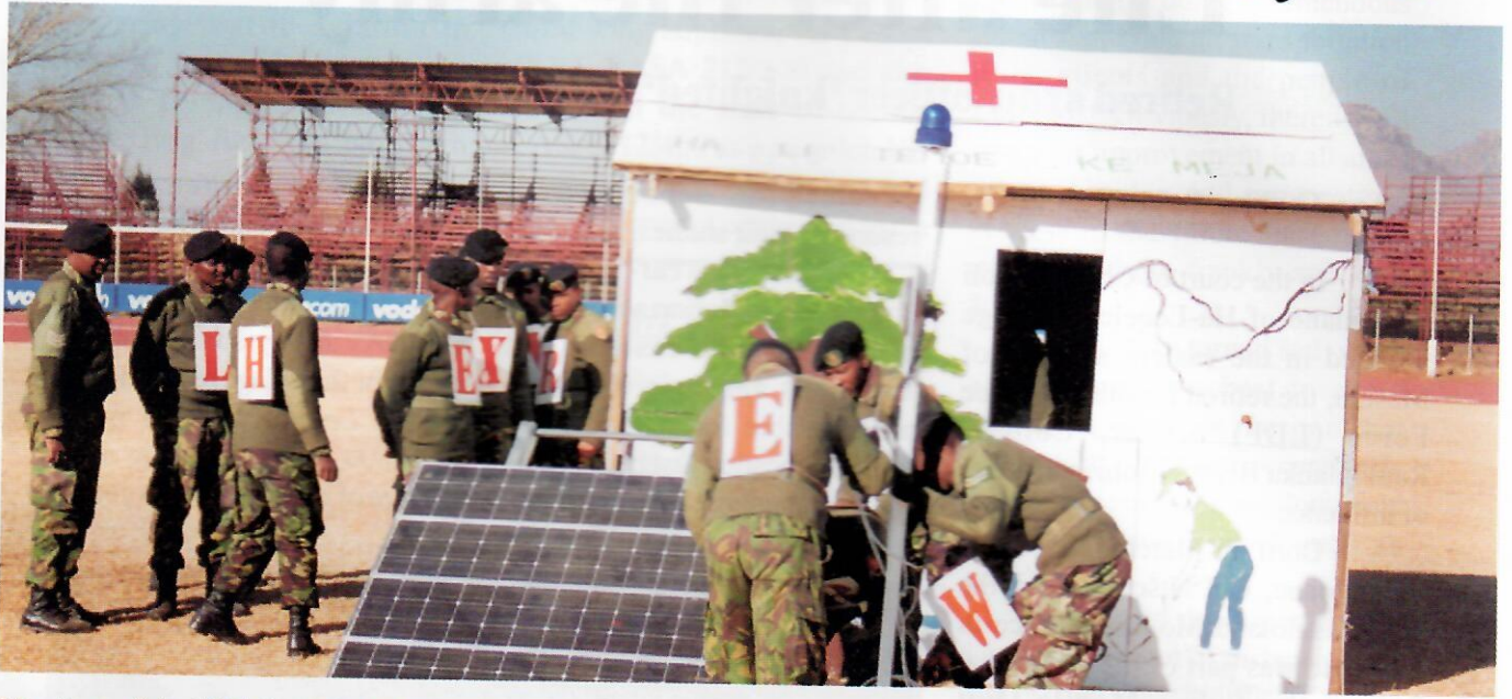
Members of the LDF Combat Engineers installing solar panel to generate power for a makeshift community health facility.
